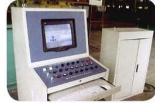
控制柜 Control cabinet
