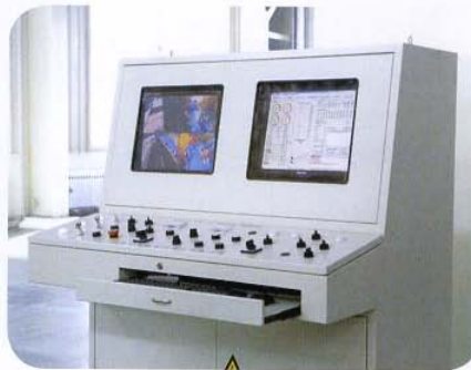
操作台 Operation station
