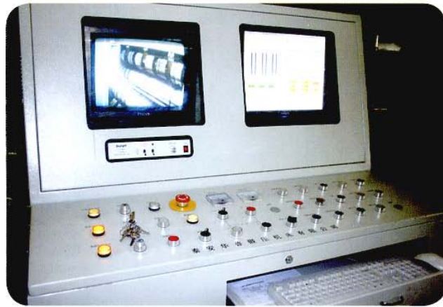
操作台 Operation station
