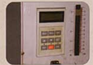
Variable speed drive control
